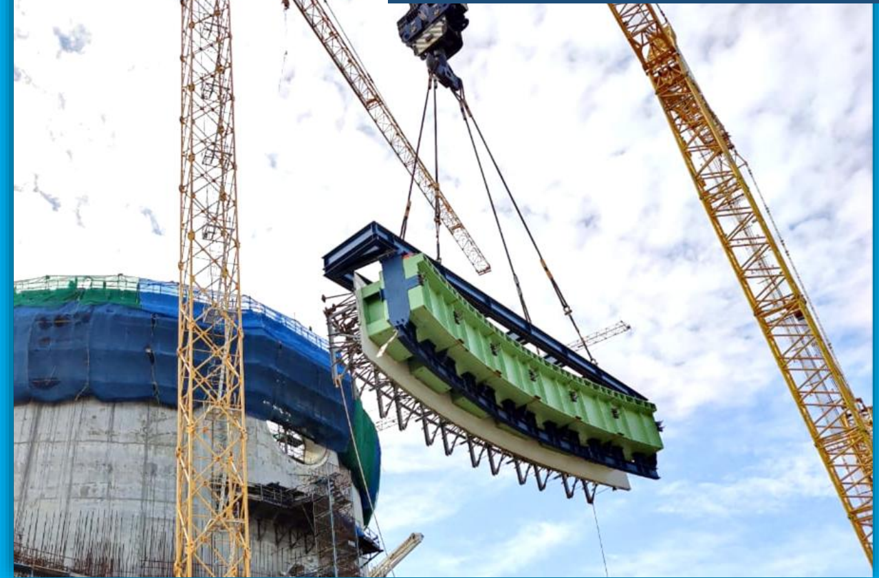
Polar Crane Brackets: KKNPP 3&4
